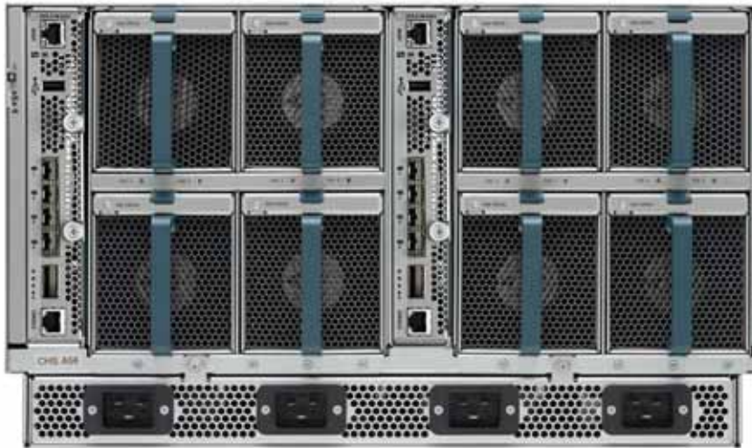
Figure 3 Cisco UCS 5108 Blade Server Chassis with Fabric Interconnects (rear view)
